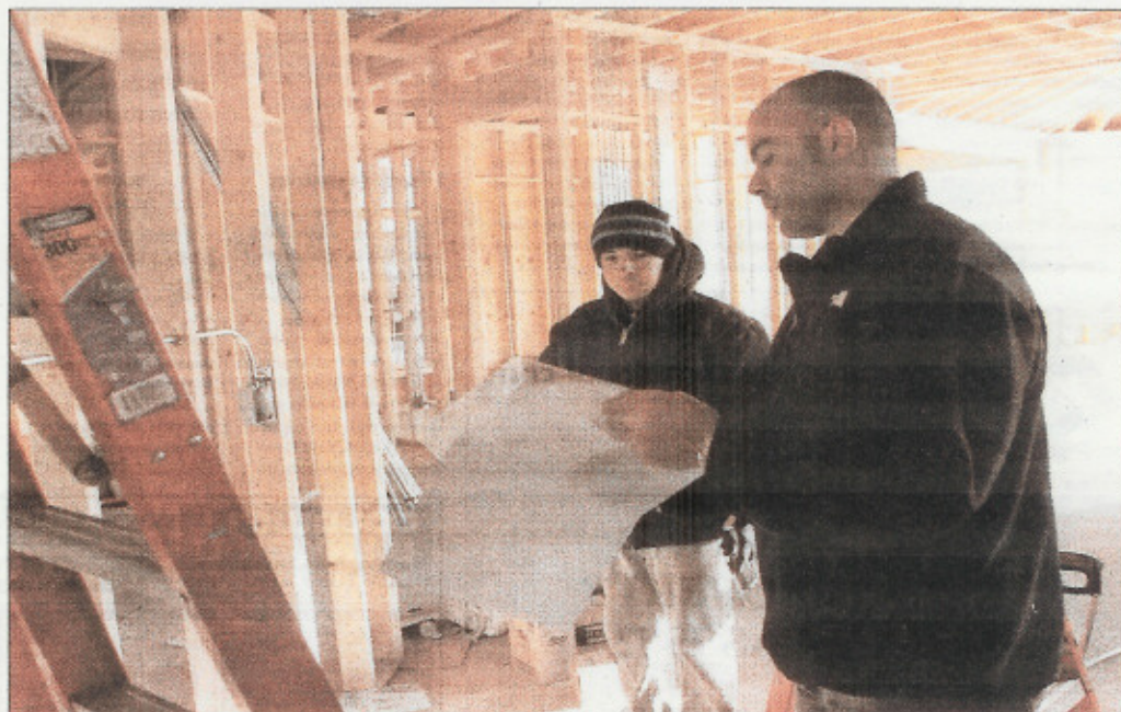
Nick DiCosola of Distinguished Dwellings of Hinsdale talks with Victor Correa of Sin-Tech Electric while working on the construction of a house in LaGrange Highlands. DiCosola builds high-value, custom homes. DOINGS PHOTO BY RENÉ EDGE
